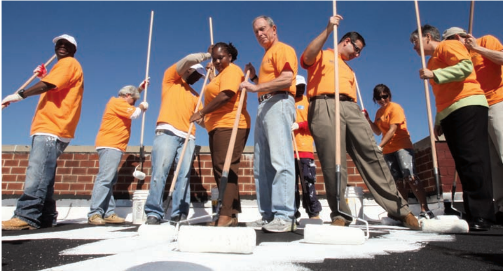
New York City Mayor Bloomberg and others participate in “NYC Cool Roofs,” reducing carbon emissions by painting rooftops white.
